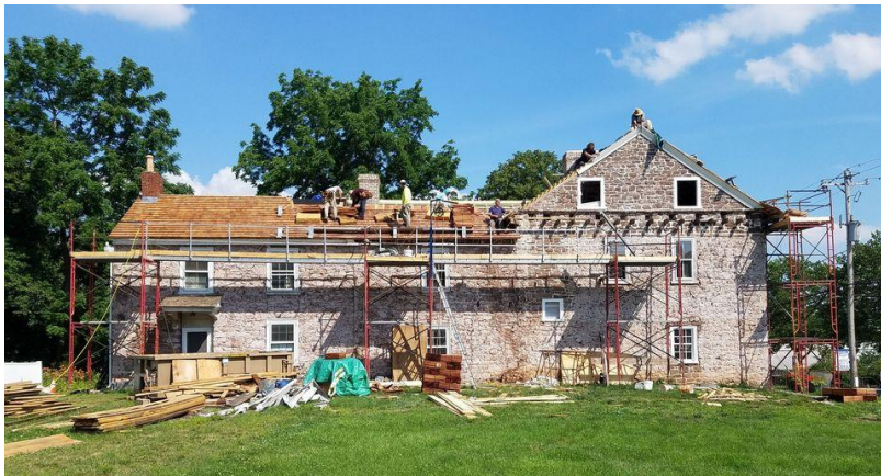
At Historic Trappe, restoration of the (First U.S.) Speaker's House, August 2023 (Facebook)
