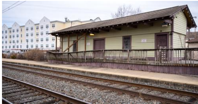
Ambler Train Station's Pre-Civil War Freight House Sits on the Crumbling "Honey Run" Culvert
