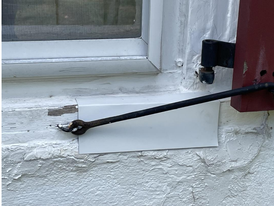
A little aluminum siding provides a temporary fix to water damage at the school
