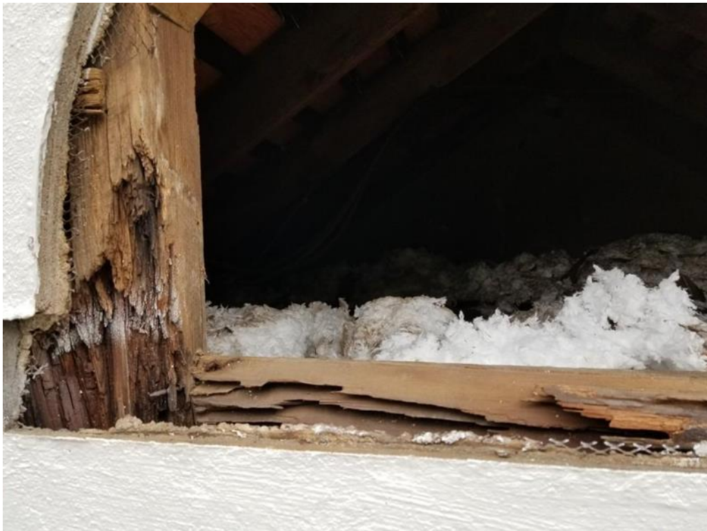
The two photos above show the vent above the rear door and the rot behind it, Nov 12, 2025. Wood from 1858?
