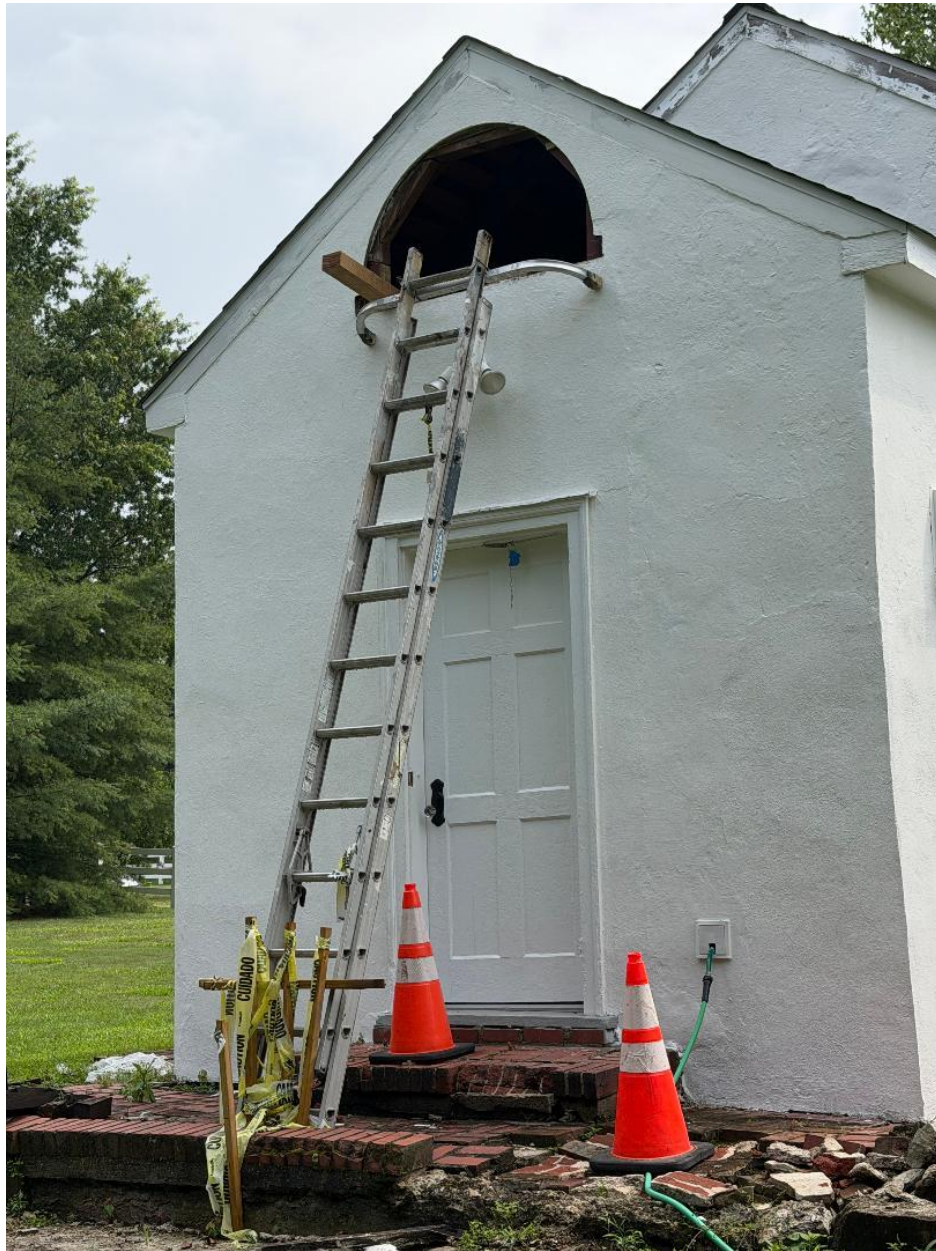
The attic vent opening, where squirrels used to enter (Photo from Barry Johnson, July 13, 2026)
