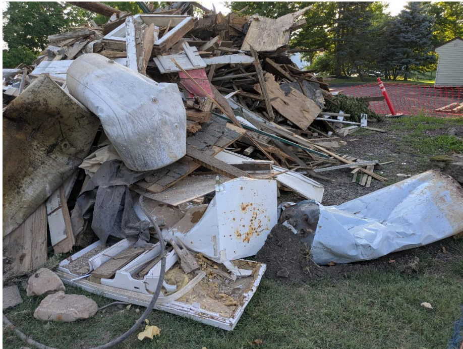
This pile contains an oil tank, a water heater, and what might be a refrigerator door.
