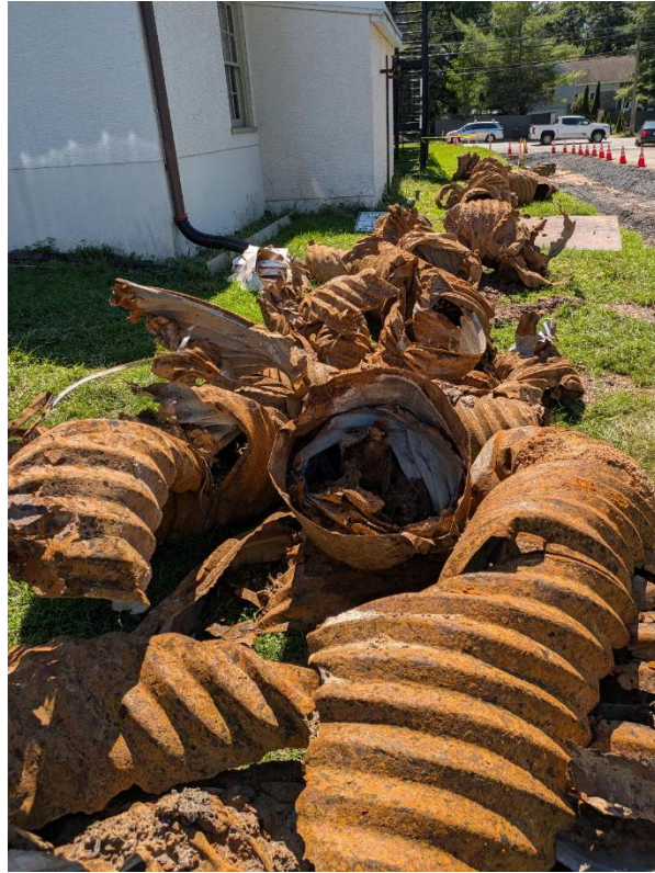
Old culverts were ripped out and left as a strange configuration.
